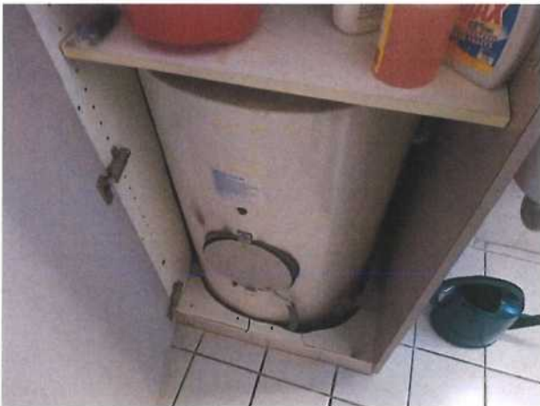
Elektroboiler 120 Liter, ca. 1990
